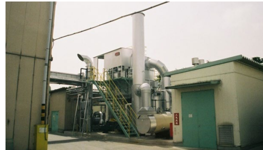
VOC abatement system in the Tochigi site
